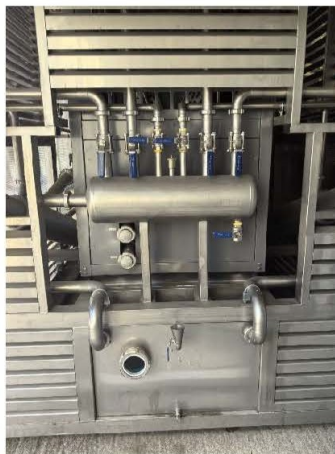
recirculating cooling water system
