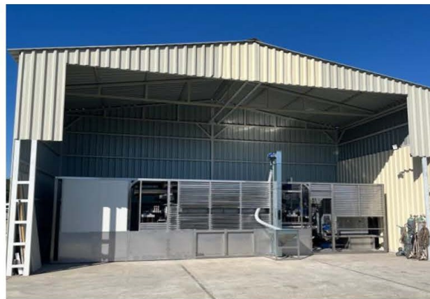
INODES installation with fifth generation plasma assisted pyrolysis system PAP
