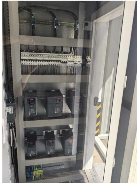
management and monitoring system
